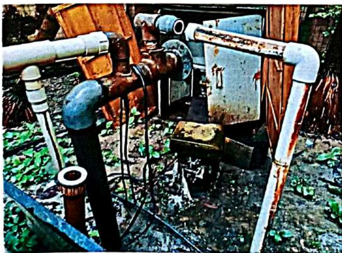
5) Bore Well (3 rd ) Non Functional
