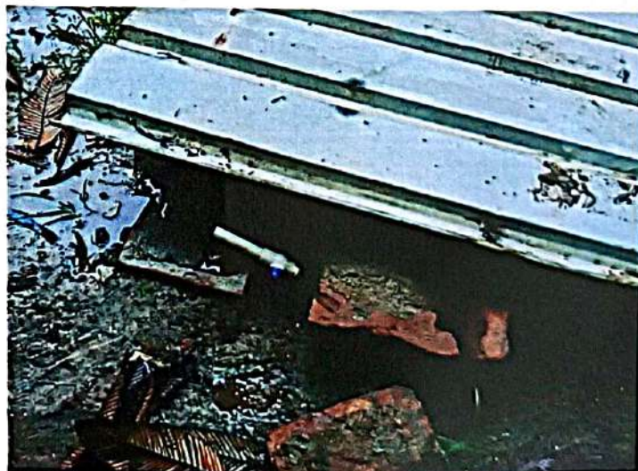
6) Bore Well (4 th ) Functional but totally cemented
