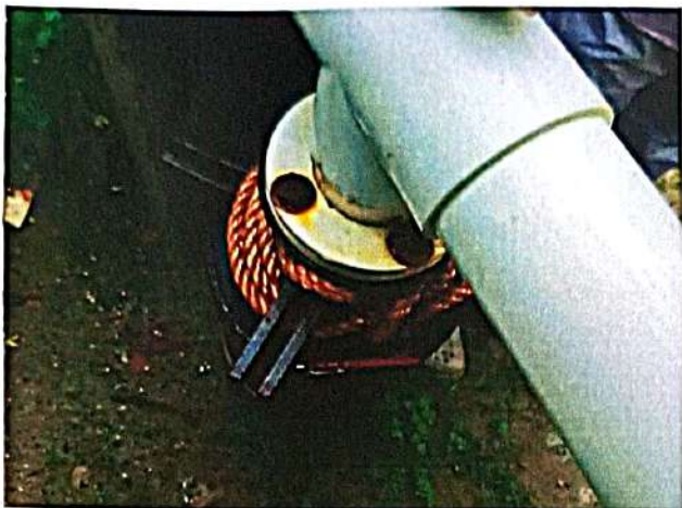
7) Bore Well (5 th ) Functional
