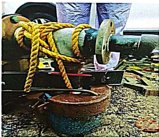
3) Bore Well (1 st ) working condition
